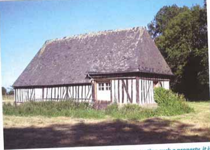
A colombage renovation project in Eure. When renovating such a property, it is important to make sure that any cement render is replaced as soon as possible
